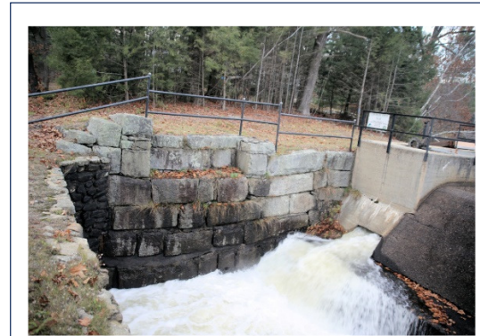
2017 photograph shows granite railroad bridge abutment and concrete dam with sluiceway open (Preservation Company).
