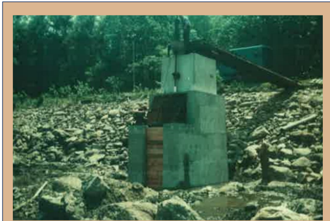
1978 drawdown inspection photo shows the concrete drop inlet and gate and stoplog bay after repairs in 1976 (NHDES).
