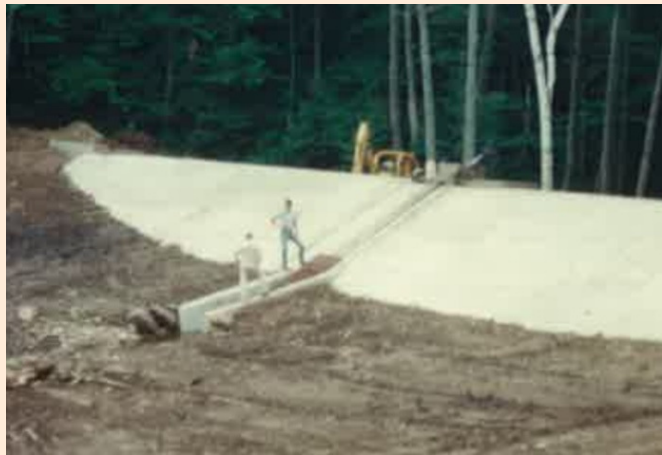
In the 1990s, the upstream face of the concrete spillway was resurfaced, and new gate stem installed (NHDES).
