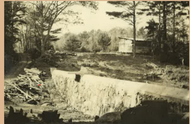
Childs Bog Dam stone downstream face. Construction took place between August and October of 1924 (NHDES).
