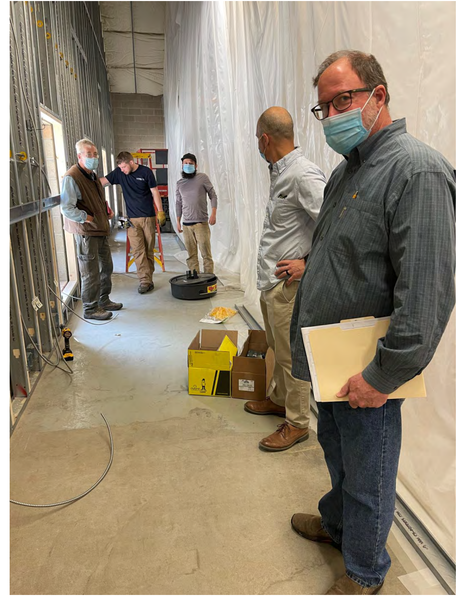
Chair of HHI's Energy Committee Doug Gline has been working hard to ensure extensive improvements (insulation, efficient heating, solar power) as part of Harrisville Designs renovations to the Cheshire Mill Complex.
