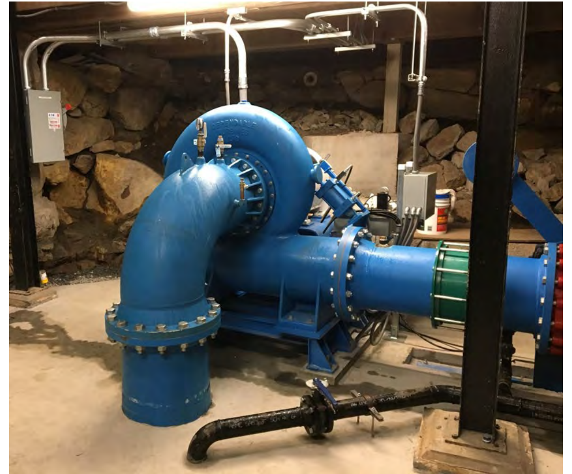
38 kW “Francis Type” Hydro Turbine drives an induction generator, installed in Oct/Nov 2018.
