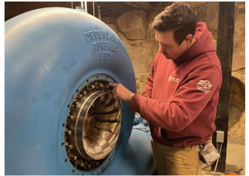
A contractor conducts the annual cleaning of the turbine to remove debris and ensure efficient operation.
